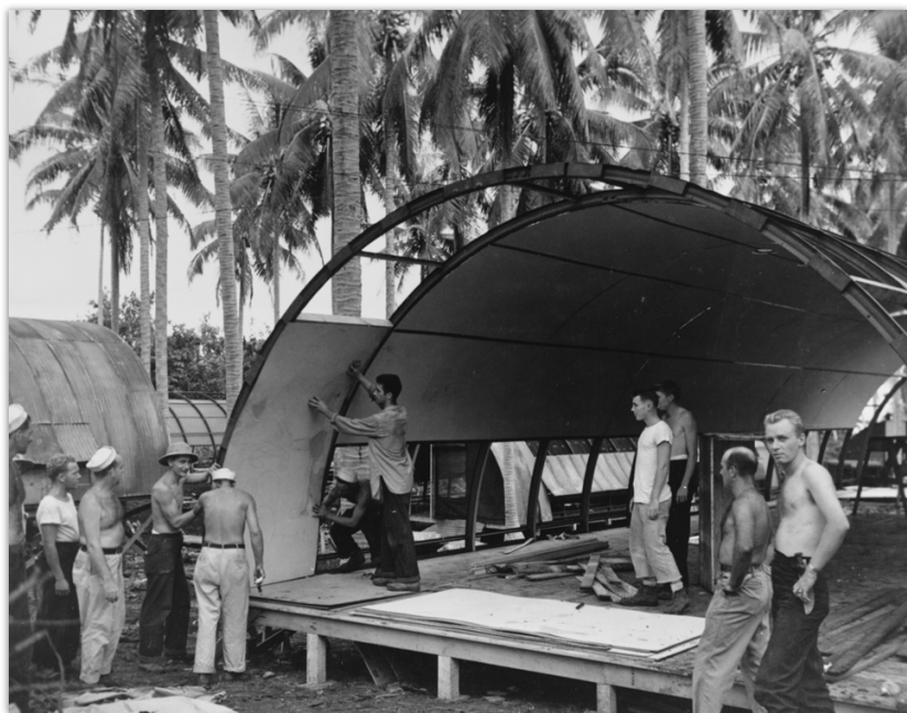
33rd Construction Battalion constructing Quonset hut pilots' quarters on one of the Russell Islands, 10 November 1943 (NHHC 80-G-56521).
